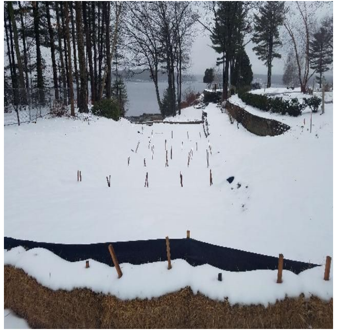
Fig 2: Slope at Gundalow landing/east side of the Bay. Viewing west. (02-06-20).
