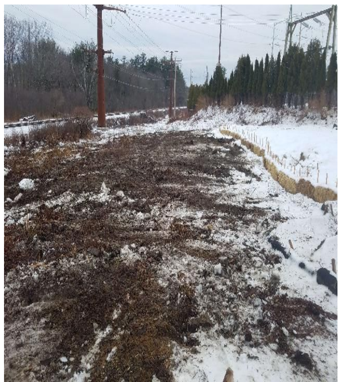
Fig 8: Crew continues to remove timber matted access road for Strs. 1 and 2. Viewing south. (02-10-20).
