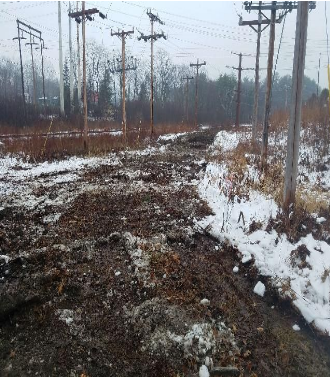
Fig 11: Timber mats have been removed from Madbury substation to Str. 3. Viewing south. (02-11-20).
