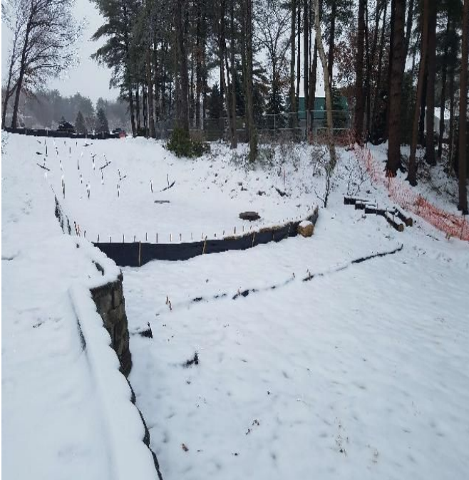
Fig 5: Slope at Gundalow landing/east side of the Bay. Viewing east. (02-07-20).
