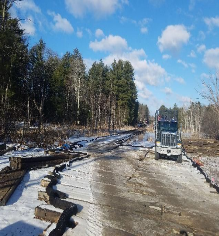
Fig 13: Crew building access road from Str. 116 to Str. 114. Through wetlands NW11 and NW13. Viewing north. (02-12-20).
