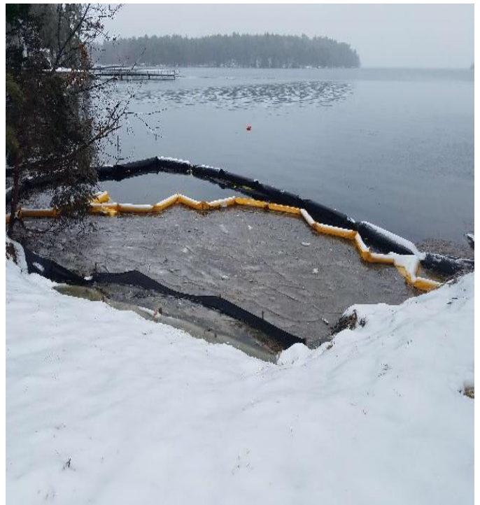
Fig 4: Turbidity barrier in intertidal zone at Gundalow landing/east side of the Bay. Viewing southwest. (02-07-20).
