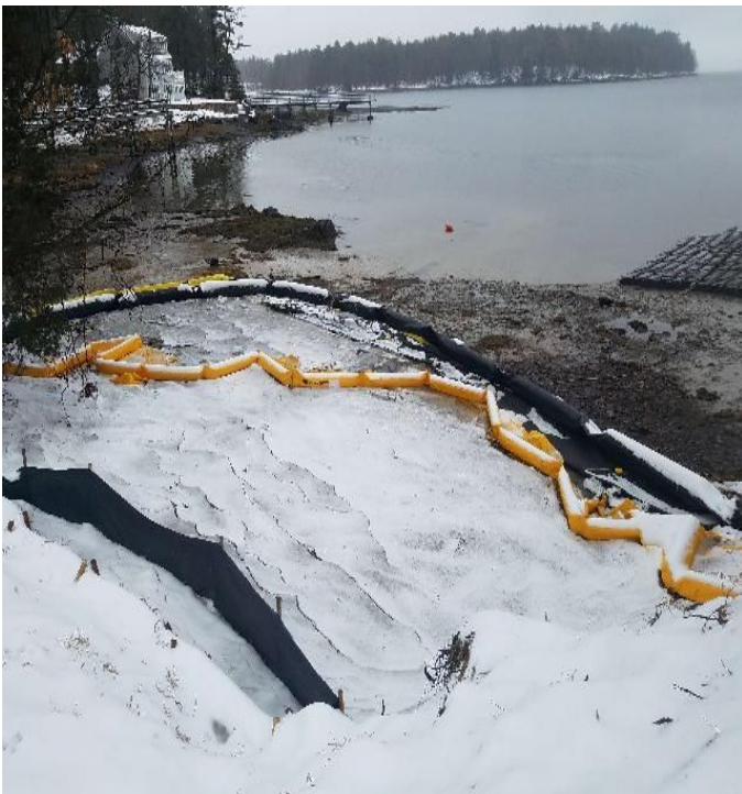
Fig 3: Turbidity barrier in intertidal zone at Gundalow landing/east side of the Bay. Viewing southwest. (02-06-20).
